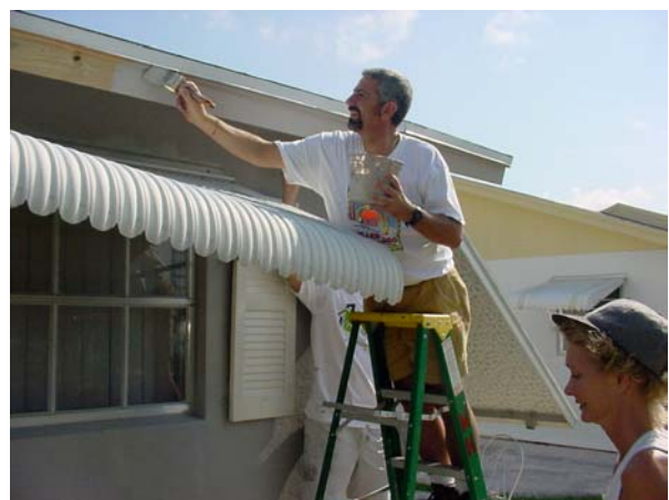
Peter Aquart demonstrates his painting acumen at the Hedrick Brothers Construction/ASCE House.
